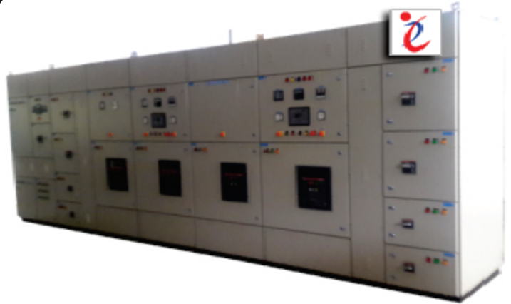
AMF Panel & DG Synchronization Panels
