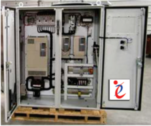
PLC - Automation Control Panels
