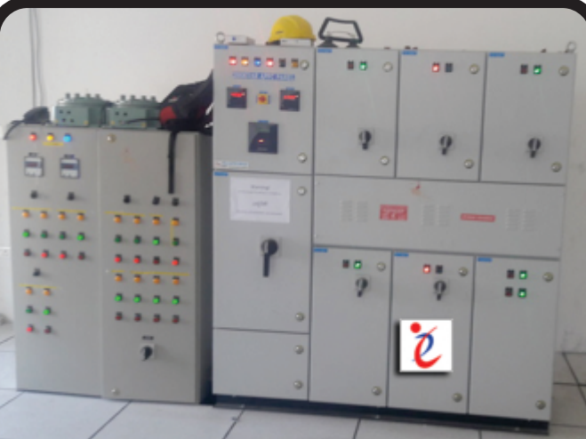
Automatic Power Factor Correction Panels - APFC Panels
