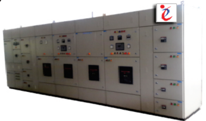
AMF Panel & DG Synchronization Panels
