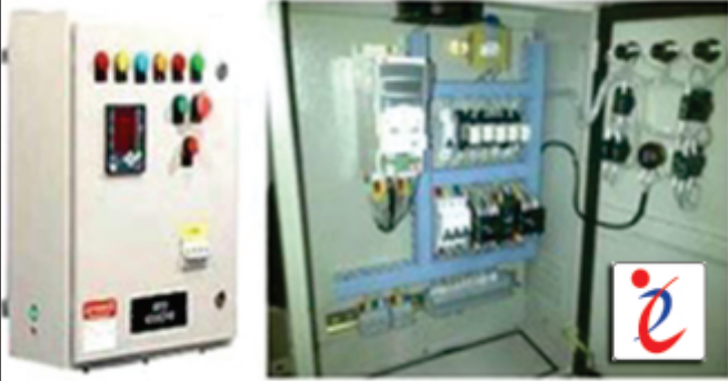
AHU Air handling Units Panels
